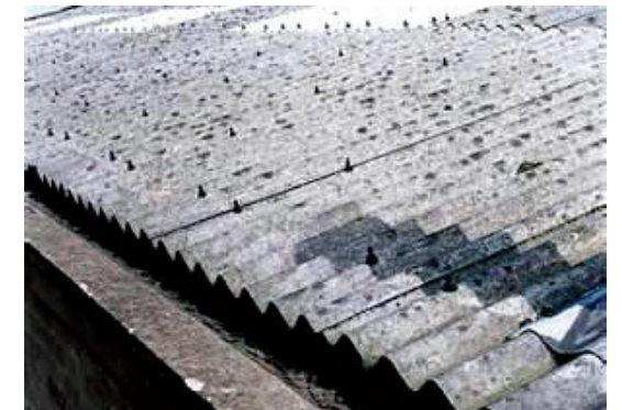
ASBESTOS ROOFING & BOARDS
