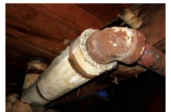
ASBESTOS LAGGING & INSULATION
