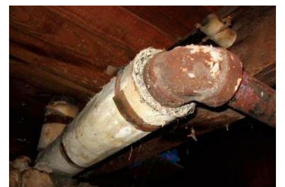
ASBESTOS LAGGING & INSULATION
